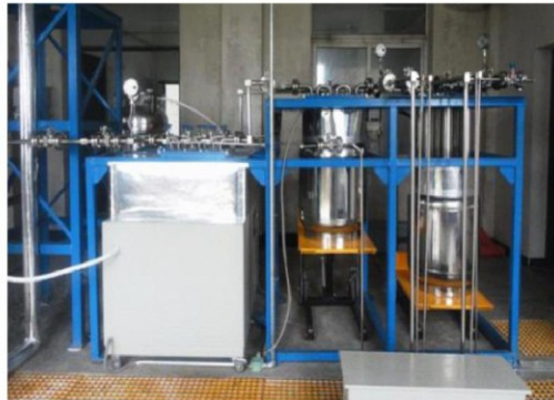
Germane Cryogenic Treatment Producing Line
